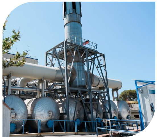
Solvent Recovery Unit (SRU) at Sessa Arunca - Italy
