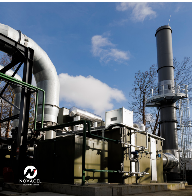
Regenerative Thermal Oxidizer (RTO) at Déville-Lès-Rouen - France
