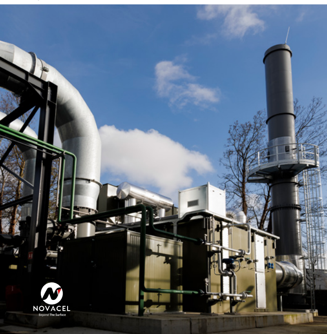
Regenerative Thermal Oxidizer (RTO) at Déville-Lès-Rouen - France
