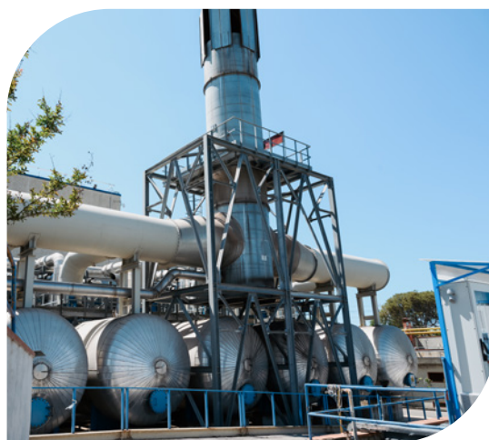
Solvent Recovery Unit (SRU) at Sessa Arunca - Italy
